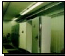
Motor control center
