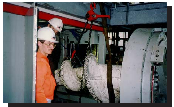
Service technicians assisting with mechanical change-out of major drive assembly in Grafton, Ohio.
