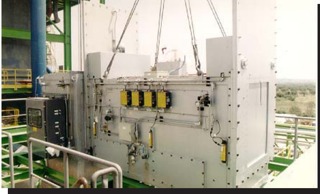
Complete airlock assembly with nitrogen purge and oxygen sampling system.
