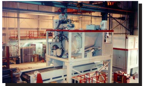
Dual auger shredder with horizontal steel belt conveyor assembly.
